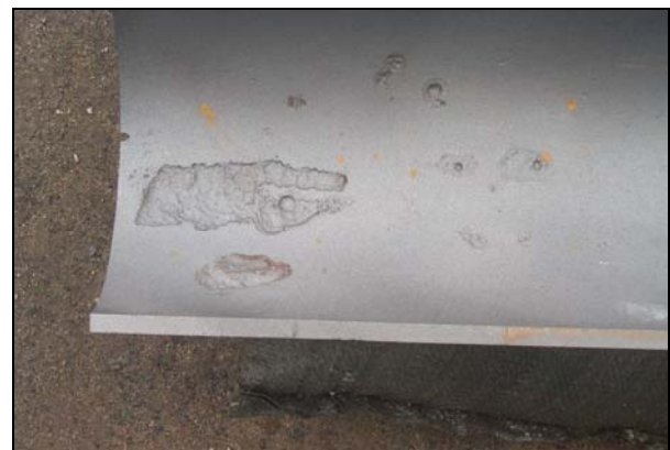
Pitting corrosion on interior of the same cast iron pipe
