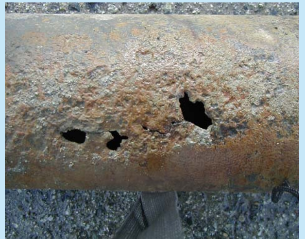
Corrosion on a ductile iron distribution water main
