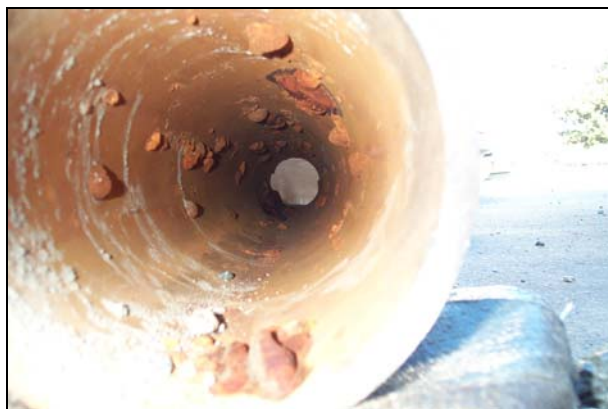
Corrosion nodules on interior of cast iron water main
