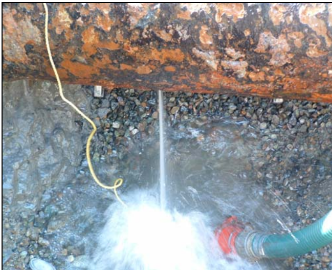
Leak in a steel water transmission pipeline
