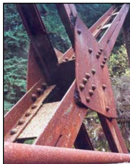
Corrosion Product Wedging of Riveted Bridge Superstructure
