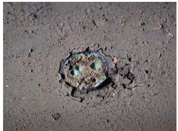
Cluster of corrosion pits observed beneath a tubercule on the internal diameter surface of a copper water distribution tube.
