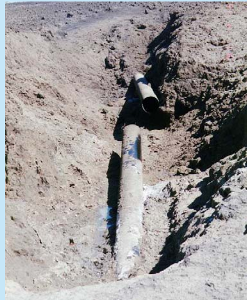
High-pressure gas transmission pipeline that failed due to stress corrosion cracking.
