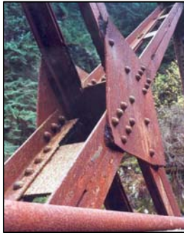
Corrosion Product Wedging of Riveted Bridge Superstructure
