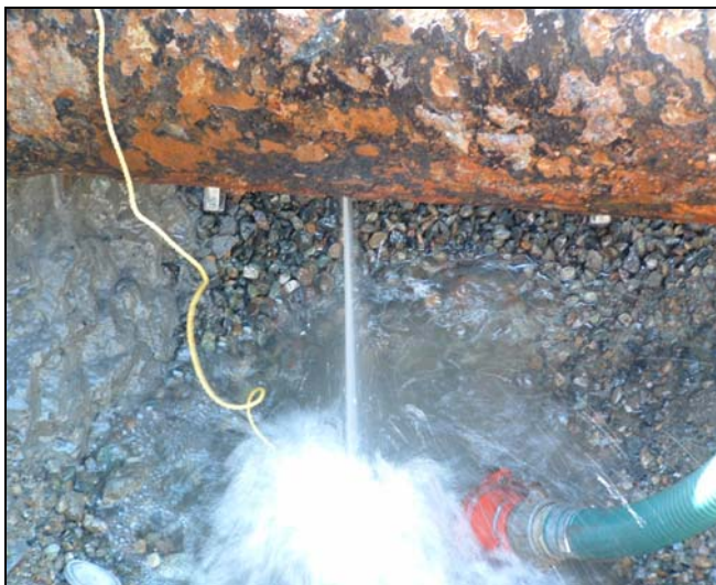
Leak in a steel water transmission pipeline
