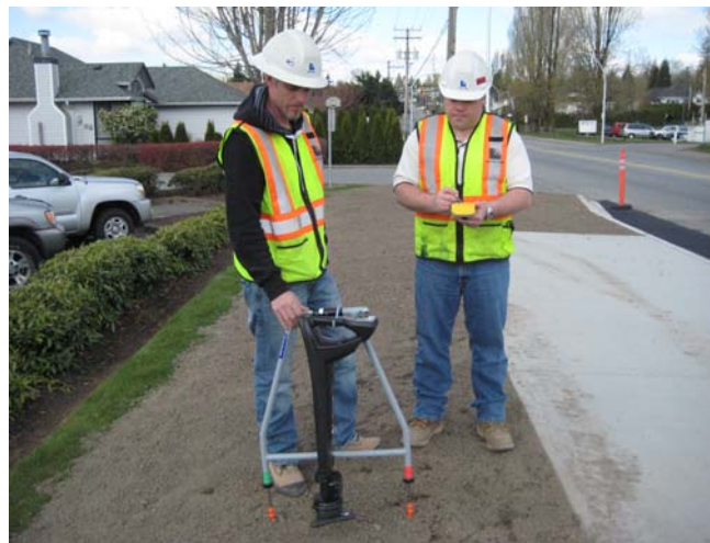
Pipeline Current Mapper & A-frame
