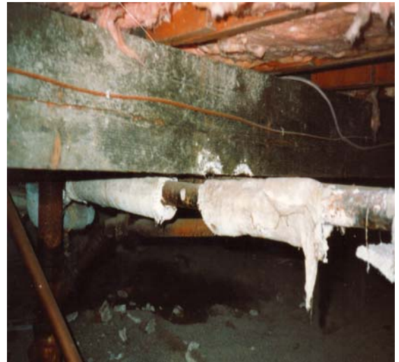
Asbestos Pipe Insulation
