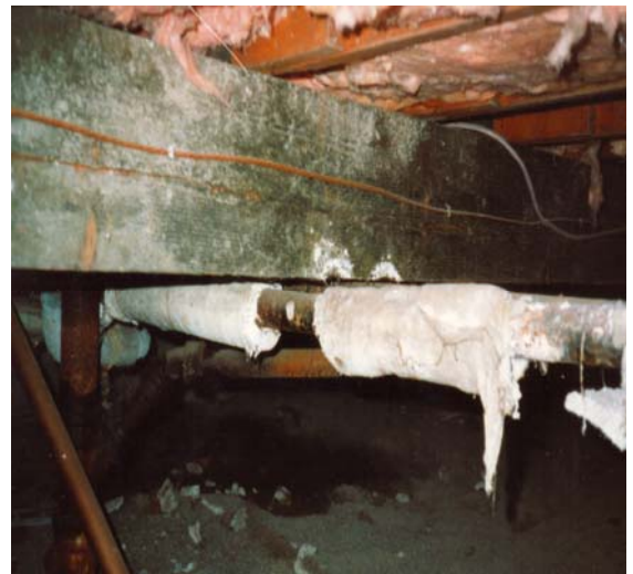
Asbestos Pipe Insulation
