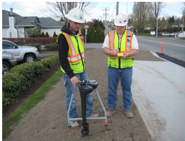
Pipeline Current Mapper & A-frame
