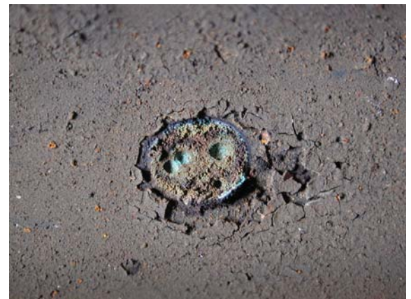
Cluster of corrosion pits observed beneath a tubercle on the internal diameter surface of a copper water distribution tube.
